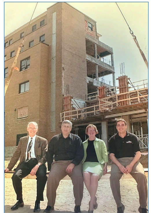
Pictured above in 2004 against the backdrop of a construction project to transform St. Joseph's Hospital into a long-term care home are John Quinlan, Director on the Foundation board, Romeo Cercone, former CEO of St. Joseph's Hospital, Eleanor Maslin, SJLCB Administrator, and Chris Friel, Mayor of Brantford at the time of construction.
